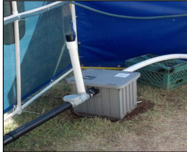
Wastewater Connection with Grease Trap
